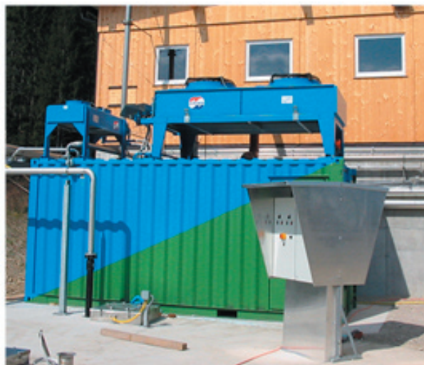
Figure 2, Installed biogas CHP module (150kWel/ 183kWth ) from "etaone holding" company (Picture: MUT company)
