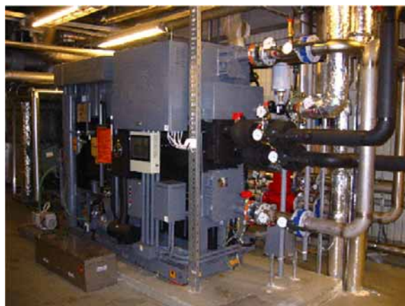
The Microturbine and Chiller Installation at Statoil, Stavanger
