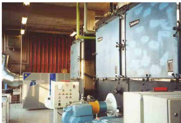
Two T-100 CHP Units installed in Heating Station West at Copenhagen Airport
